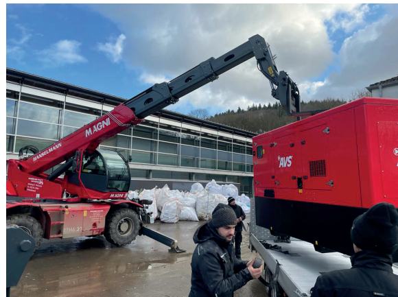
Provision of essential infrastructure, including power generators
